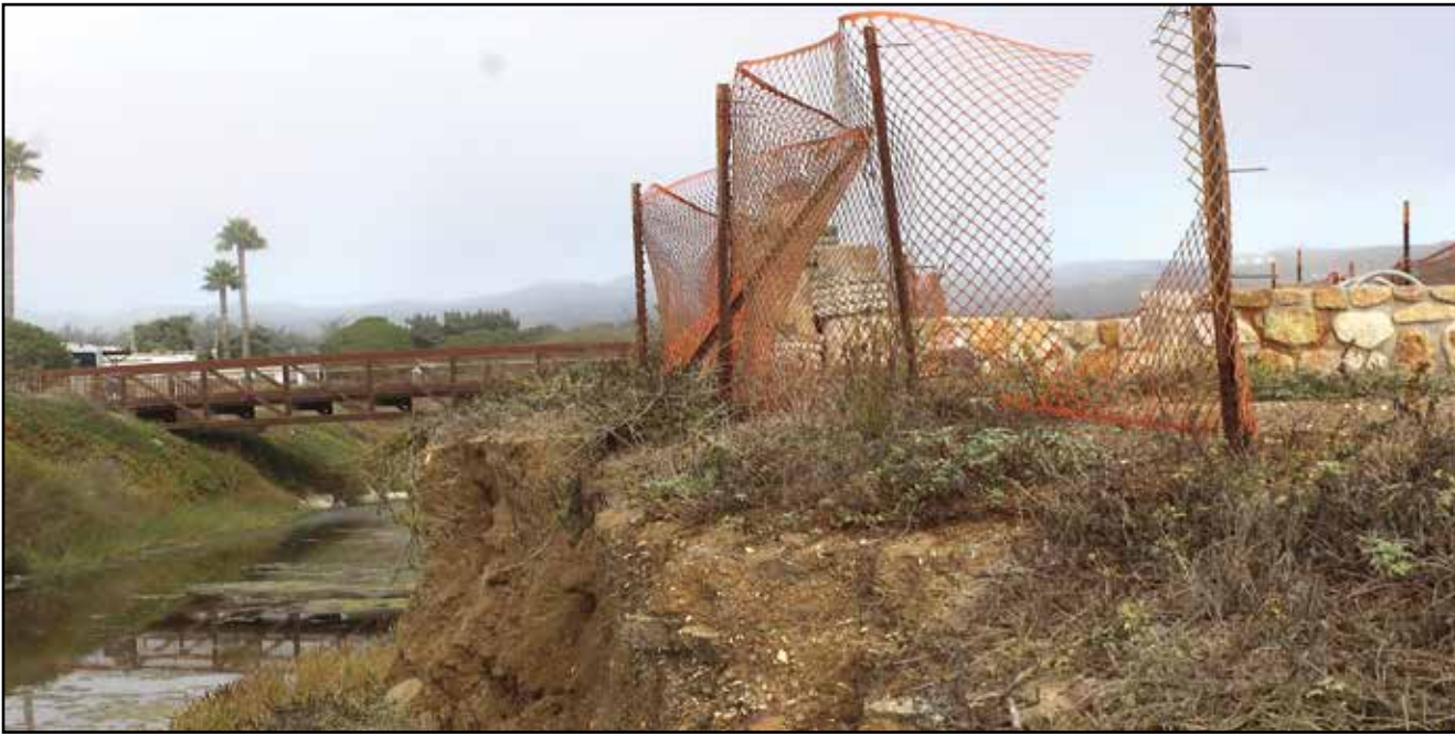
Erosion on the Harborwalk.
