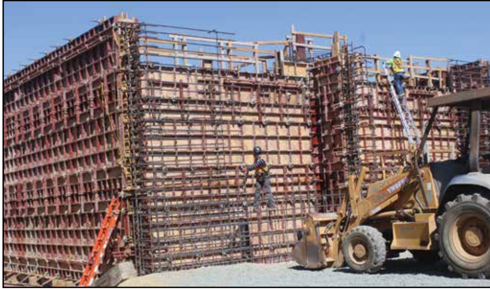
Workers fashion the rebar cage of one of two bio-reactors. The final grade of the plant site will be 10 feet higher than now leaving just a few feet of the tanks above ground; but that won't happen until after both concrete tanks have been poured, cured and filled with water to check for leaks.
