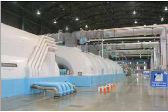
Photo shows the main generators at the Diablo Canyon Nuclear Power Plant. A hiccup in the hydrogen cooling system of one of these massive generators forced the Unit 2 reactor to be shut down, even as Unit 1 is down for refueling.
