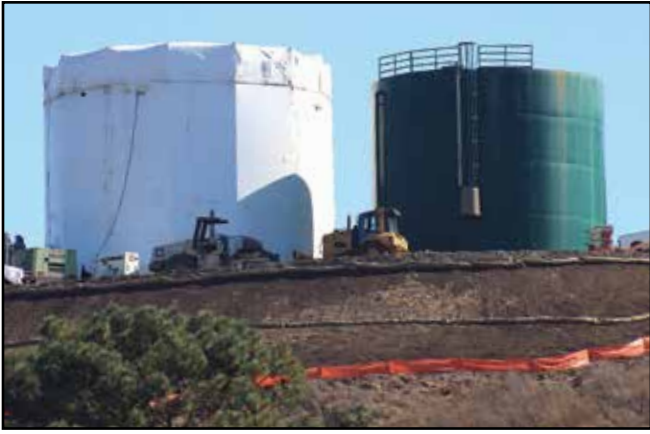
The water tank replacement and system upgrade in Cayucos will add one new 210,000-gallon storage tank and demolish and replace another tank.
