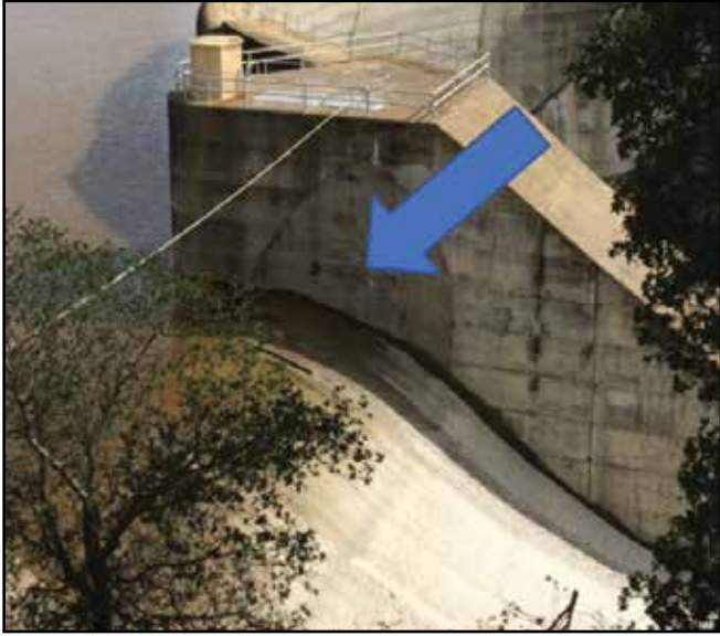
Photo shows the current spillway of the Salinas Dam. The County Flood Control District is seeking to obtain the dam from the Army Corps of Engineers, who built it in 1941. The blue arrow points to where spillway gates might be installed to greatly raise the capacity of Santa Margarita Lake. Photo courtesy SLO County
