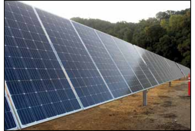
The County has finished much of the construction on a 1.2 megawatt solar farm off Oklahoma Avenue that will help power some 12 County facilities, including the various jails, saving over $5 million over 20 years. Photo by Neil Farrell
