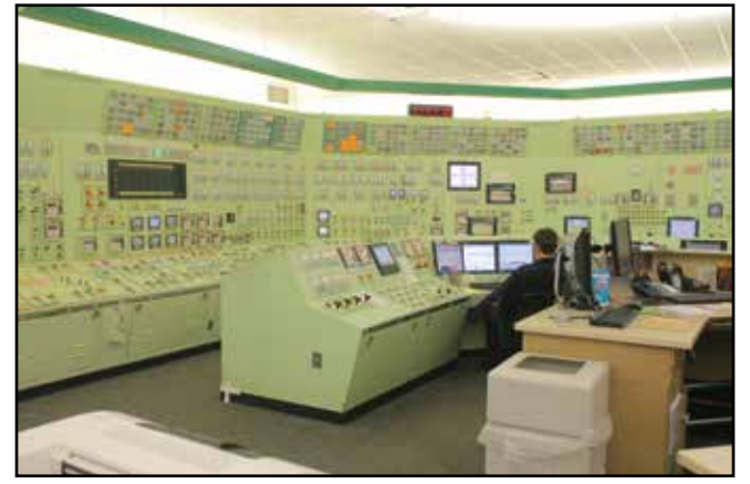
Here’s a peek inside the control room at the Diablo Canyon Nuclear Power Plant.
