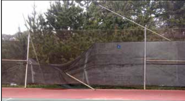
Photo shows the damaged fence around the tennis courts at Monte Young Park.
