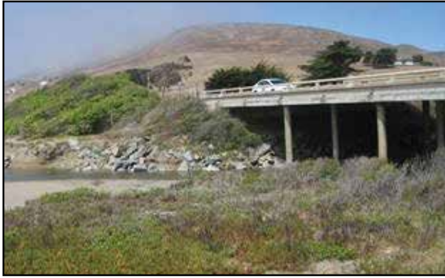
The Morro Bay-Cayucos Connector Bike Way will have to span the 150-180 feet of Toro Creek with a standalone bridge hefty enough to carry the weight of a maintenance truck. File photo
