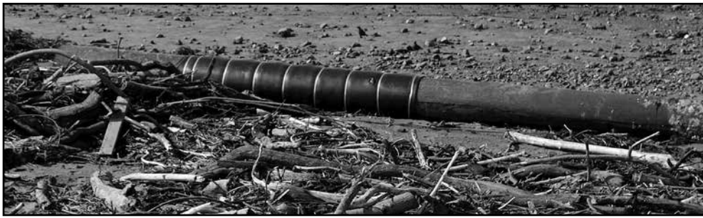
One of the Cayucos Pier piles lies at the mouth of Cayucos Creek, ripped out of the ground by massive waves.
