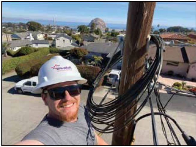
Astound's construction manager for the Morro Bay project, Justin Hunt, takes a selfie from atop a utility pole while stringing fiber optic cable in Morro Bay. Submitted photo
