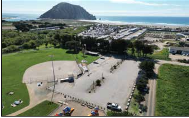
This photo taken with a drone, shows the layout of the Lila Keiser Park, with the parking lot in the center adjacent to the park's west softball diamond. The parking lot is being repaired and repaved plus handicap accessible improvements. Photo courtesy City of Morro Bay
