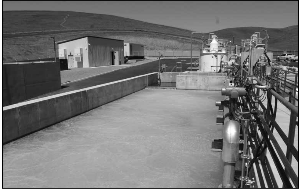
August 2022 photo of the new treatment plant's activated sludge digesters before microbes were introduced and the plant started taking in sewage. These ponds were set back when sludge brought in to activate the plant died and the process had to be repeated.
