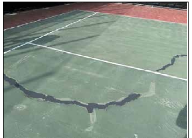
Photo shows some of the cracks in the surface of the Monte Young Park tennis courts before City maintenance crew resurfaced them.
