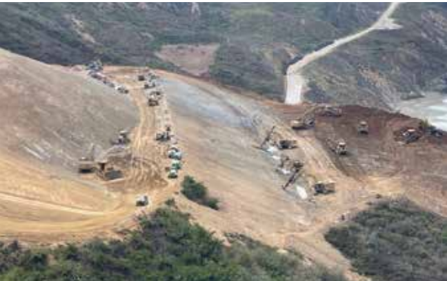
Overhead photo shows the massive Regents Slide scar on Hwy 1. The hillside above the roadway slipped out in January 2024 and obliterated the highway. Caltrans has been working since then to stabilize the slide and eventually rebuild the roadway. Photo courtesy Caltrans
