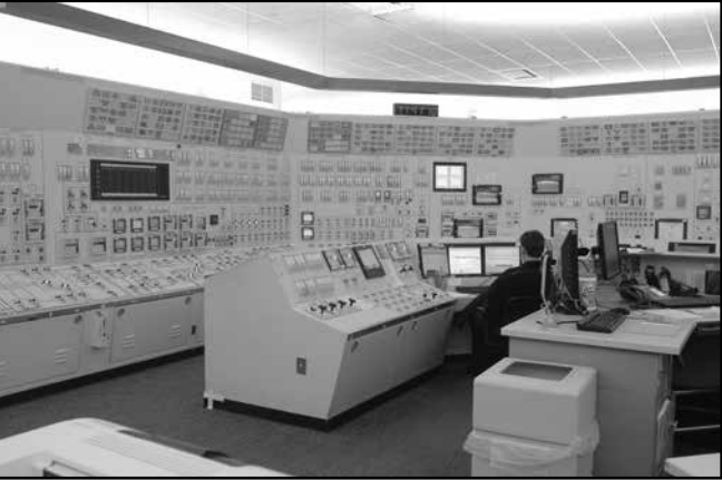
A look inside the control of the Diablo Canyon Nuclear Power Plant. Photo by Neil Farrell
