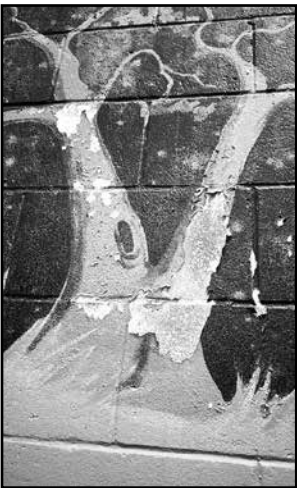
Paint on parts of the mural is peeling off to the cement. Photo submitted
