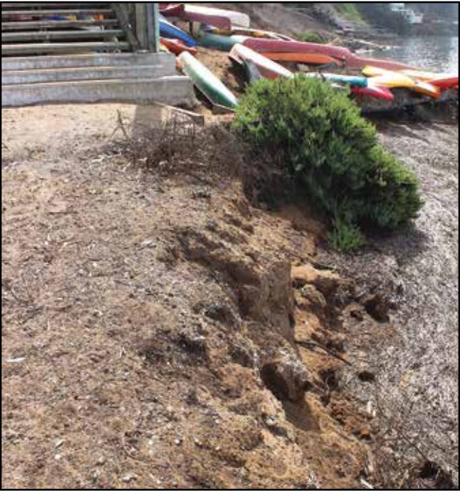
Looking north from the beach at Bayshore Bluffs shows how close erosion has come to the base of the stairway.
