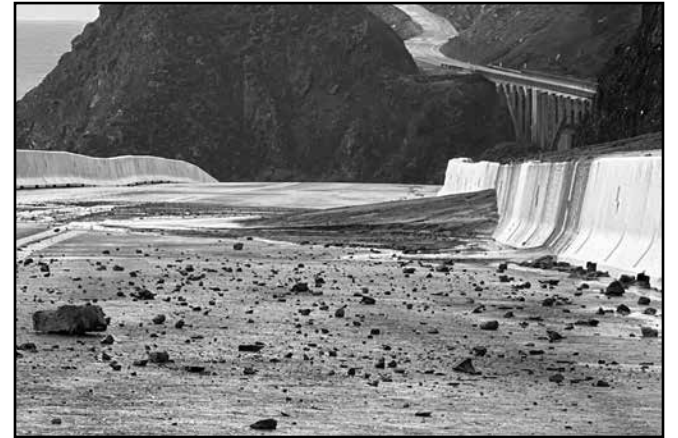
Rocks, mud and debris overtopped a concrete barrier on the northbound shoulder of Hwy 1 at Regent's Slide, forcing Caltrans to close the highway again, after reopening it in mid-January after nearly two years being closed. Photo courtesy Caltrans
