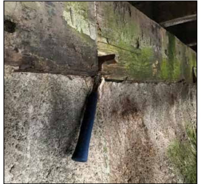
Photo from the support structure for the Morro Bay Fishermen's Wharf and a deteriorated timber cap. Photo courtesy M.B. Harbor Dept.
