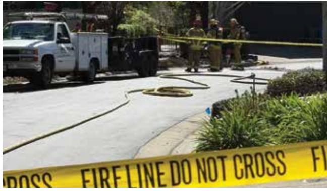
CAL FIRE caution tape marks the perimeter set up after excavation workers ruptured a gas main in Avila Beach. Photo courtesy CAL FIRE
