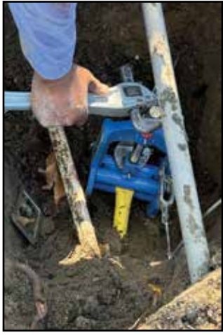
A gasman repairs a rupture in a 1-inch gas main in Avila Beach that caused the evacuation of about 100 people. Photo courtesy CAL FIRE
