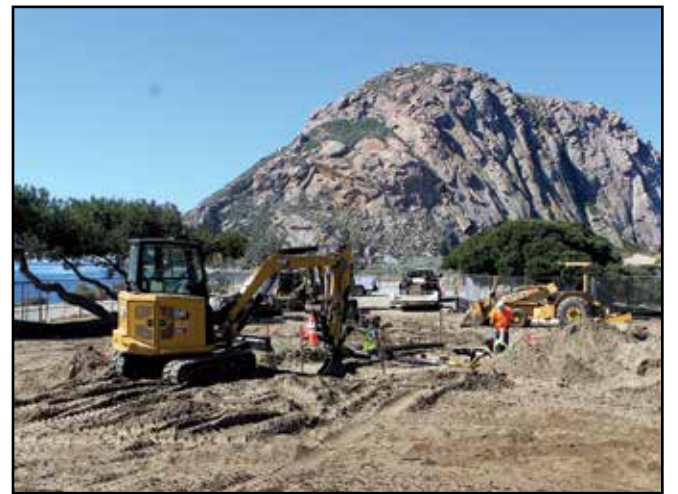
Work has begun on Phase 1 of the Coleman Park Project. Photo by Neil Farrell
