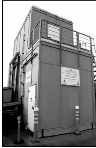
This industrial ice maker was installed in 2007 and is an integral part of the fishing industry, and now under the new lease for Morro Bay Seafood Co., LLC. Photo by Neil Farrell
