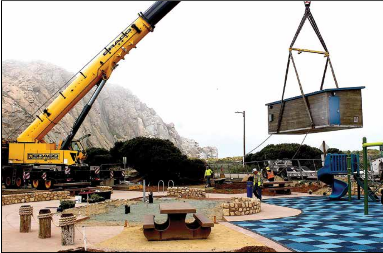
Workers with J Bruce Kies, Const., CXT Precast Concrete Products and Bragg Crane Service lift and drop into place a pre-fabricated restroom at Coleman Park in Morro Bay. The new restroom marked the completion of Phase-1 of the Coleman Park Improvements Project was nearly finished.
