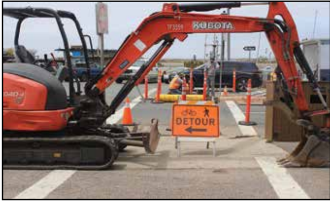
Workers with Rob Reynolds, Const., work underground to repair a break in the sewer line that services a row of buildings on Front Street. Photo by Neil Farrell
