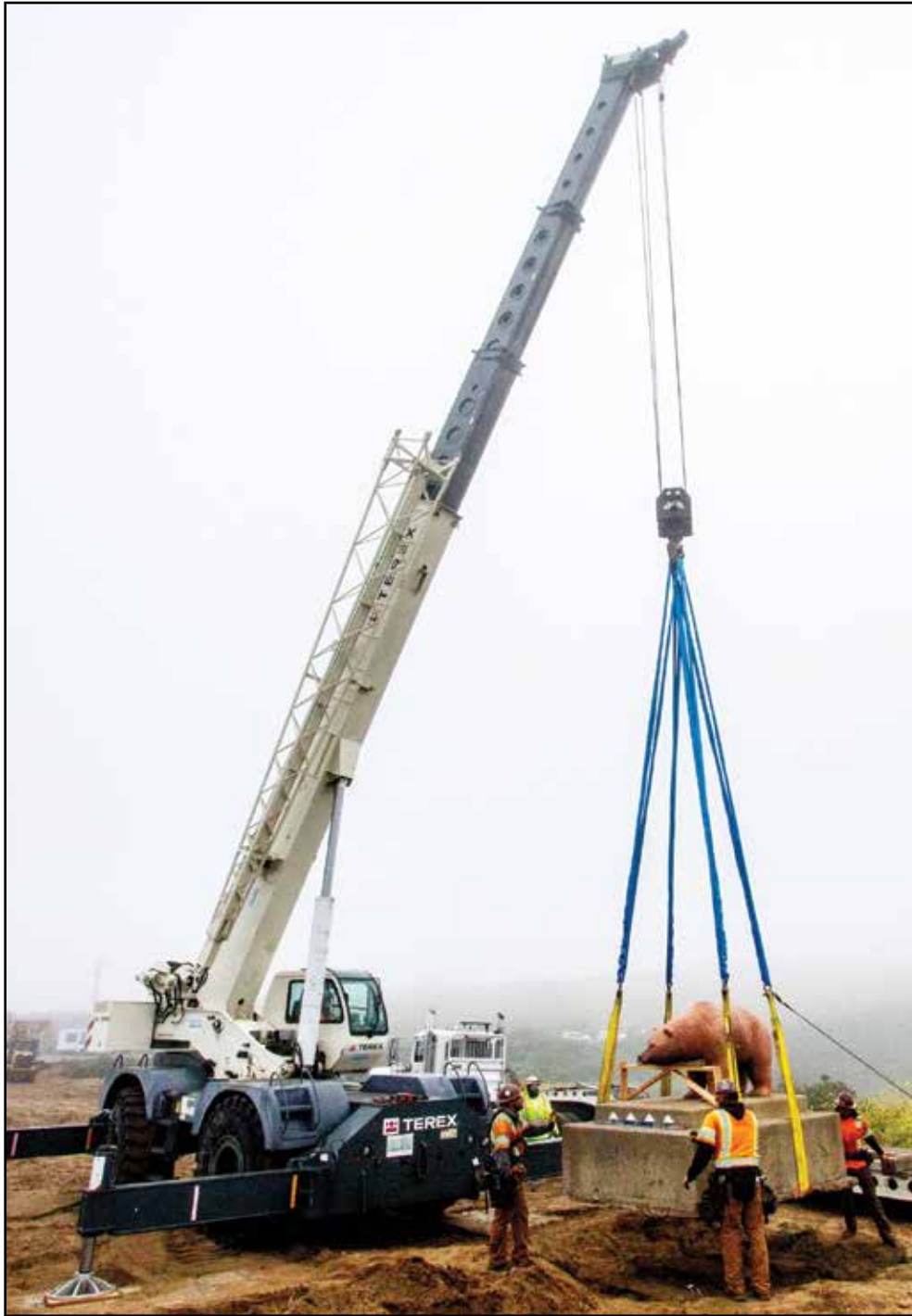
A bear statue that has become a favorite of visitors and locals alike was moved on June 1 to allow for the replacement of the South Bay Bridge in Los Osos. Often dressed up for holidays and other occasions, the bear will be back in action when the project is completed.
