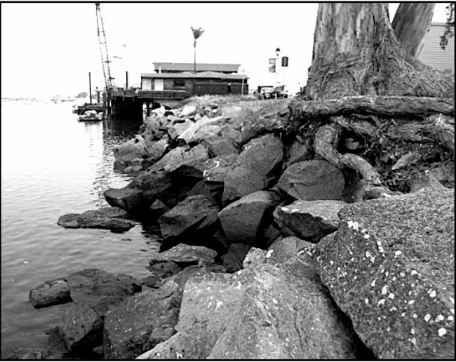
Photo shows the falling revetment along the Harborwalk as it heads towards Tidelands Park and how it is undermining a tree. City photo was put in, closing off the north entrance. The extensive sand dunes that exist today filled in quickly.
