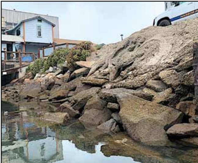
Photo shows the revetment in front of the Harbor Office with concrete slab pieces used to shore it up in the past, now falling towards the water. City photo
