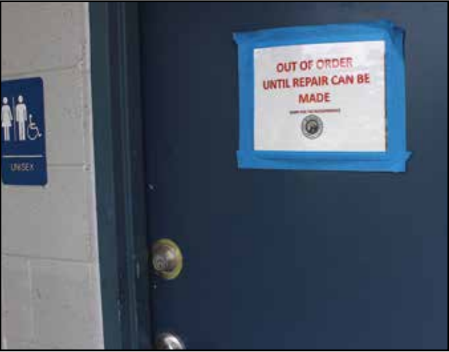
The women’s and the men’s [unisex] restrooms at Morro Bay’s City Park were closed by City officials after they were reportedly vandalized and reports came in of illicit activities taking place inside. Photo by Neil Farrell
