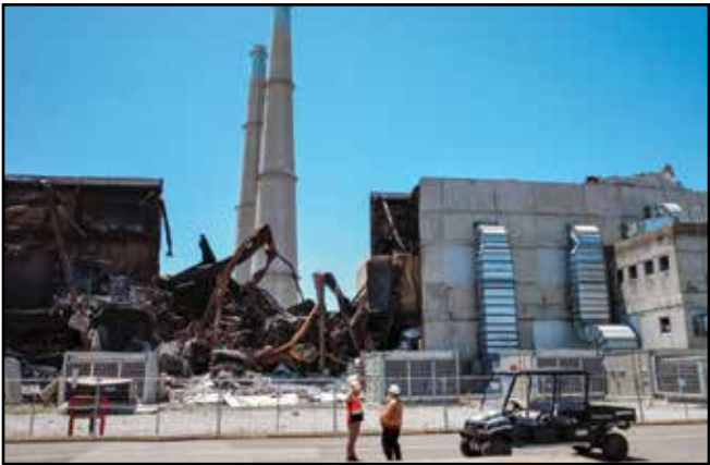
Photo from this past July shows the destroyed building where a 300-megawatt battery storage facility in Moss Landing caught fire in January 2025. Photo courtesy USEPA
