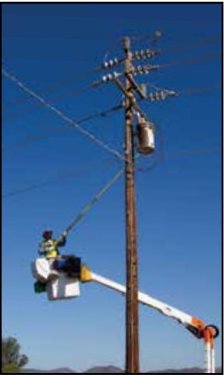
PG&E cuts power to the house for safety.
